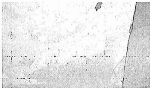
Figure 7: Disintegrating effects of mortar joints
