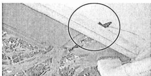
Figure 15 : Damaged gutters and ceiling board.
