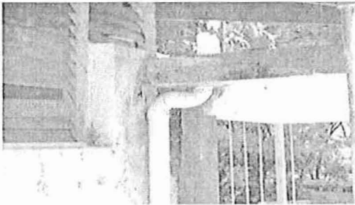
Figure 21: Dampness on wall through moisture penetration Source : Akashah et al (2006)
